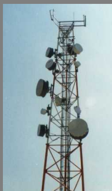
Image courtesy of Mer Telecoms
